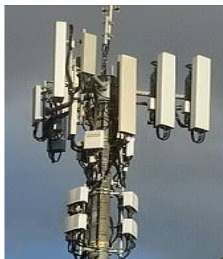
Fig :4 Cell phone antenna and its base [4]
