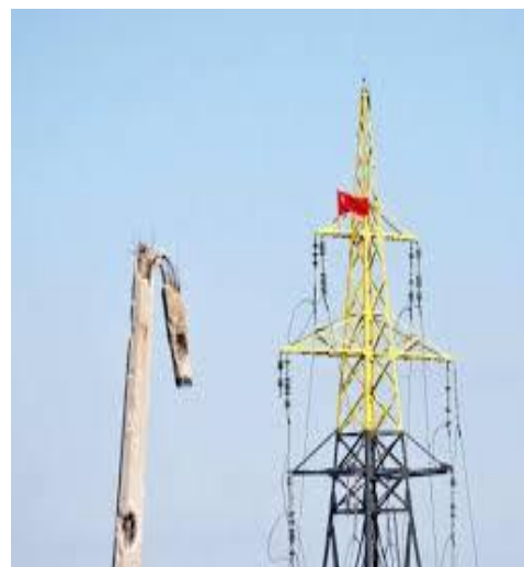
Fig :3 Cell phone antenna and its base [4]
